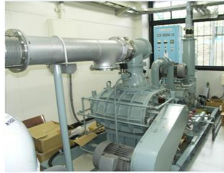
Figure 8. Vacuum exhaust pump.
