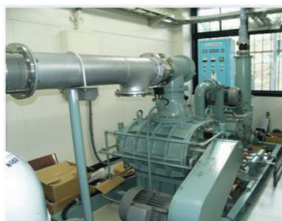
Figure 13. Vacuum exhaust pump system.
