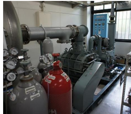
Figure 6. Photo of the vacuum pump.
